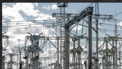
Power distribution station
