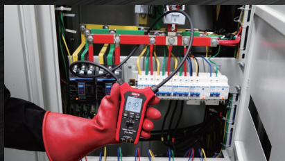
Bus bar current test
