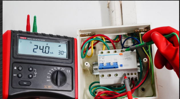
💡 Three phase RCD test
